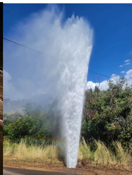
St. Moritz Water line break – 9/15/24
